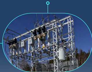
2026 Upper Coniston Substation
